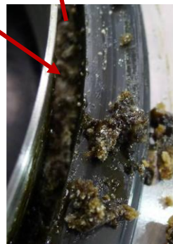
Fig 2. Uncleaned debris flange
